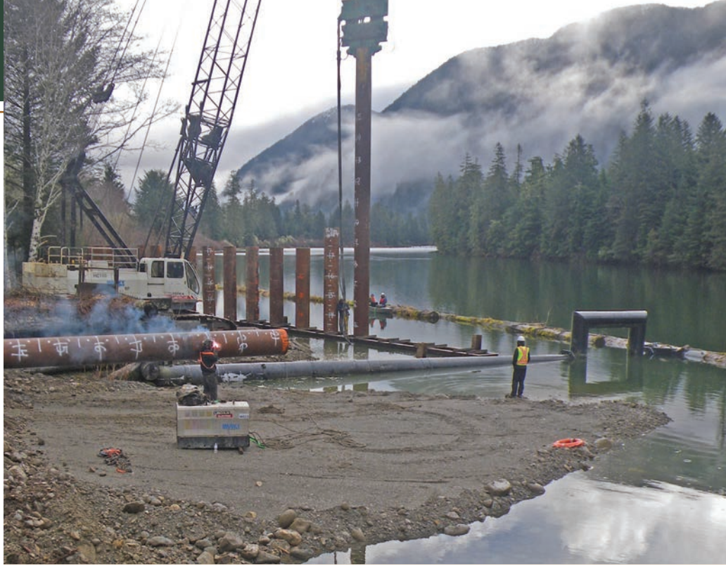
To prevent damage from debris flow damaging the central wharf in the remote BC community of Wuikinuxv (Wi-kin-oo) Nation, engineers rebuilt a debris barrier and wharf facility.
